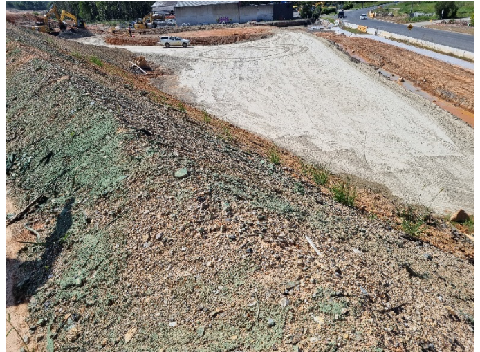
Image 2: Englands Rd, Fill 2B (Ch10900) – Looking north with Isles Dr on right, future interchange roundabout in top left
