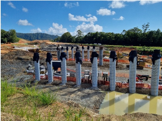
Image 7: Korora Hill Interchange, Bridge 19 (Ch20900) – Looking north across bridge piers towards Fill 17
