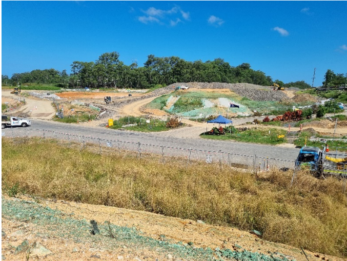
Image 1: Englands Rd, Fill 2A (Ch10800) – Looking south across Englands Rd, with soil binder application underway
