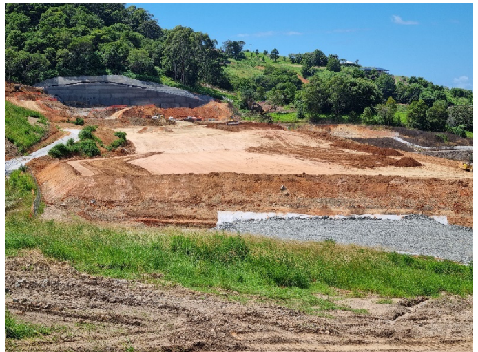
Image 4: Gatelys Rd tunnel south portal & Fill 14 (Ch18800) – Ongoing earthworks & preparation of tunnel portal
