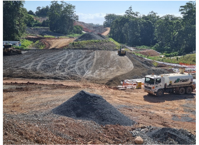
Image 6: West Korora Rd, Bridge 16 (Ch19600) – Install of piling pad in preparation for bridge construction
