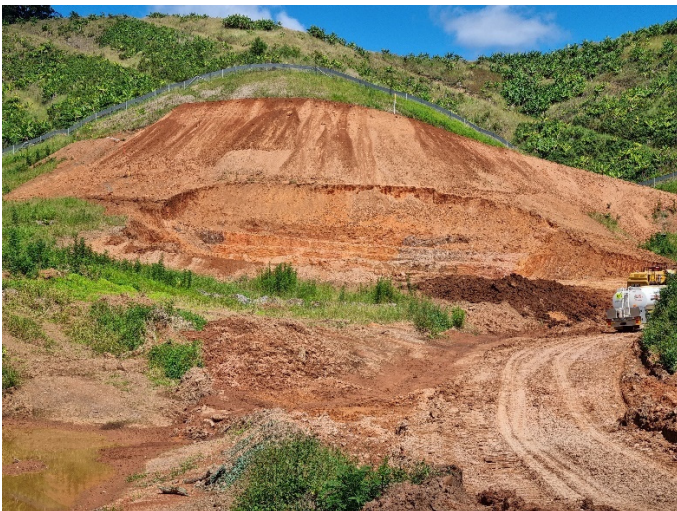
Image 3: Shephards Ln tunnel north portal (Ch17300) – Earthworks at tunnel portal following geotech works
