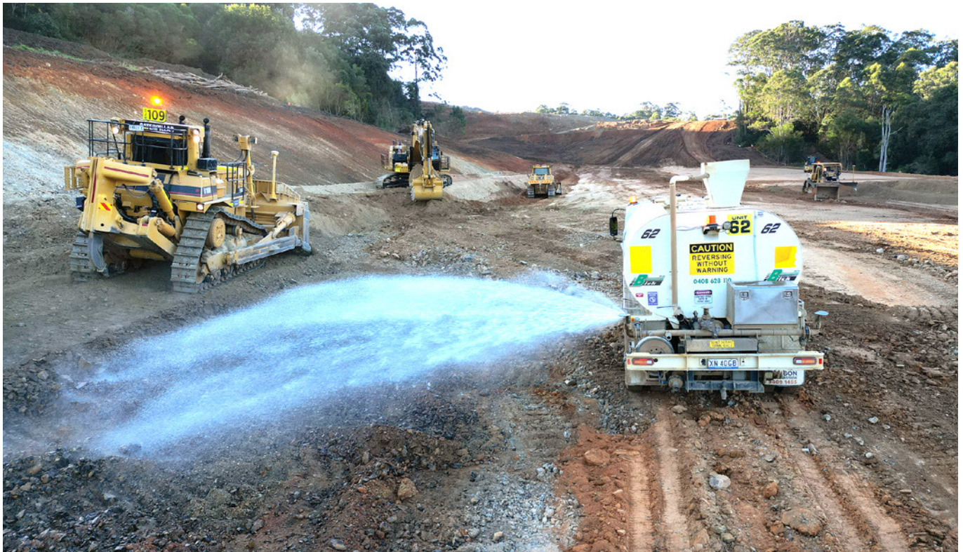
In areas where we are doing earthworks, water carts do regular runs to minimise dust on site
