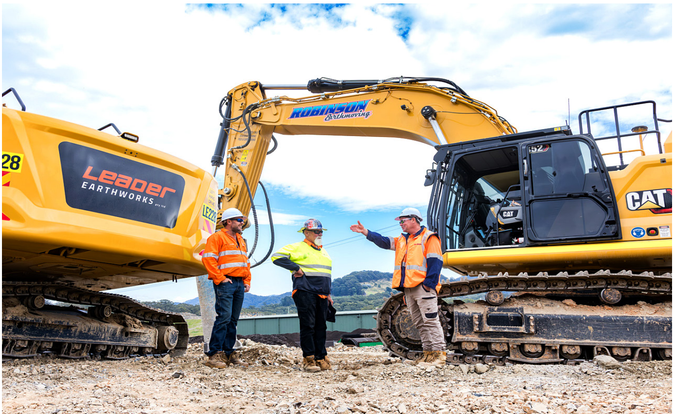
Positive communication between the Coffs Harbour bypass team on site near Englands Road
