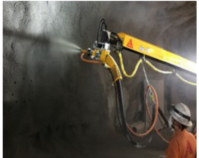
Spraying shotcrete to the walls and ceiling helps to support and stabilise the tunnel tube
