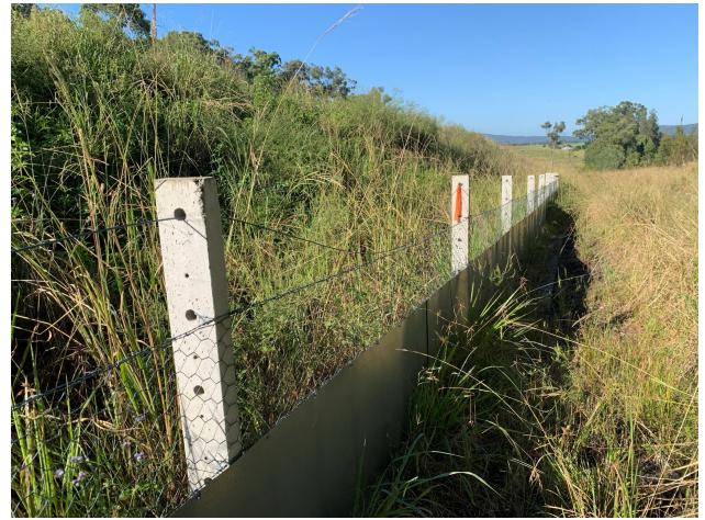
Plate 14. Damaged fauna fence identified on western side of hill on 29.03.21, was repaired same day
