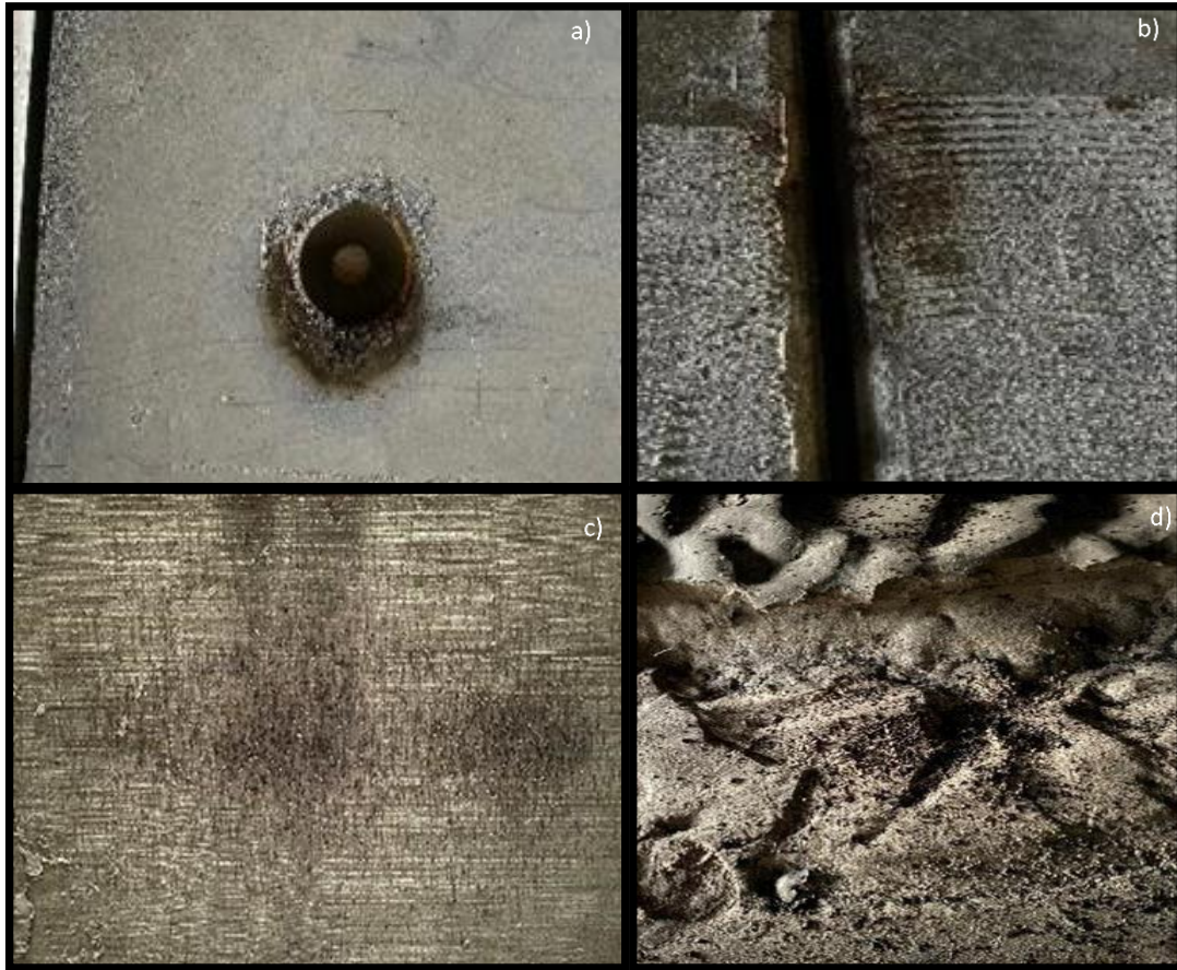
Plate 3: Microbat scuff marks around lift point (a) and culvert joints surrounded by roughened concrete (b). Microbat scat below bat boxes (c) and culvert joints (d).
