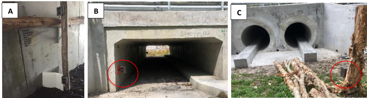
Plate 2: Typical underpass camera set-up: box culvert within sections 1-2 (A); Wardell Road box culvert – camera at each end (B); Wardell Road twin-pipe – camera at each end (C).
