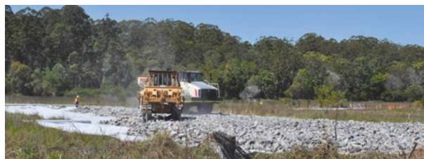
Delivery and laying of rock for an access route, south of the Kalang River
