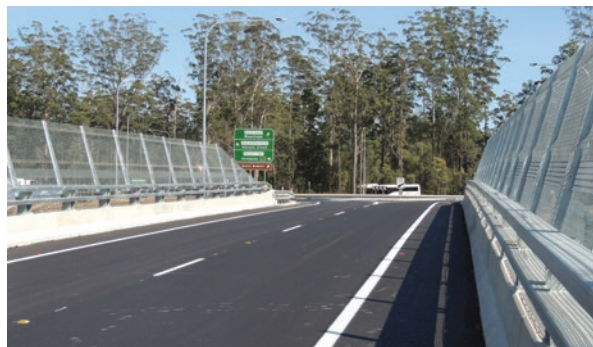
Herons Creek to Stills Road upgrade - Bago Road interchange opened to traffic on 20 September 2013
