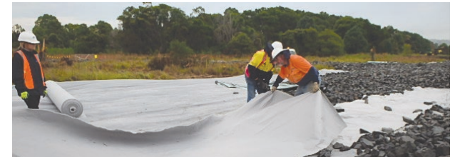
Geofabric installation prior to rock deliveries for an access route, south of the Kalang River
