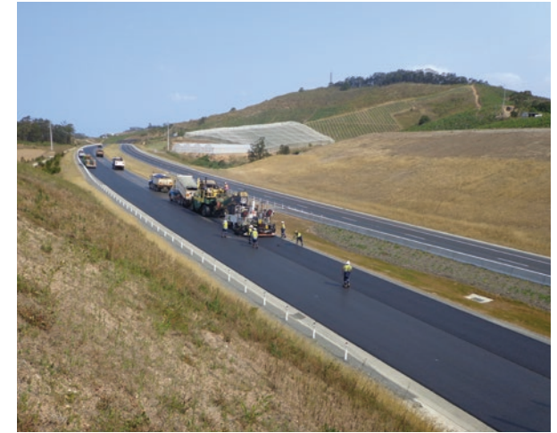
Sapphire to Woolgoolga upgrade - stone mastic asphalt being laid south of Greys Road bridge, Woolgoolga
