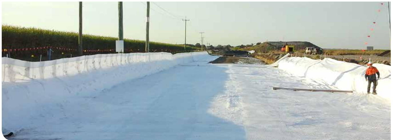
Treatment of acidic soil involved application of a lime guard layer before installation of high strength geo-fabric
